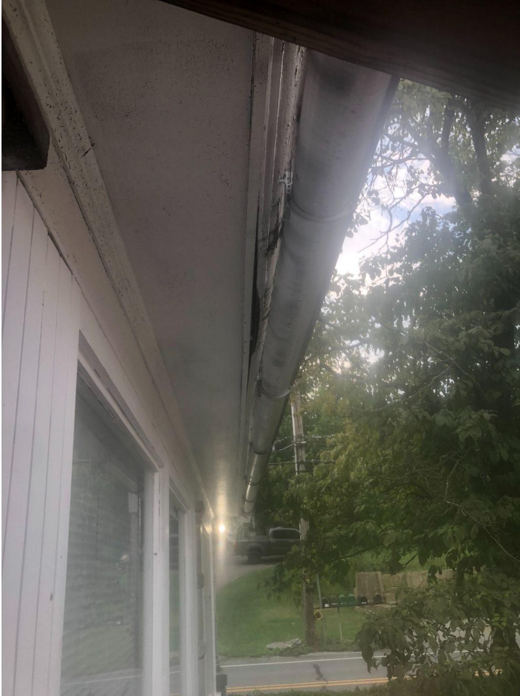
This damage is on the fascia board on the western side of the structure, approximately where the gutter attaches. This is on the roof awning level(second level)
